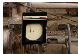
Wellhead Pressure Recording
